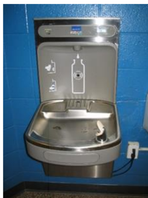
New Water Bottle Filling Stations Installed
